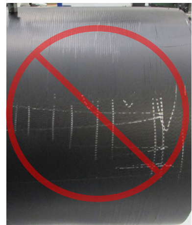
Poor scrape - markings not removed
