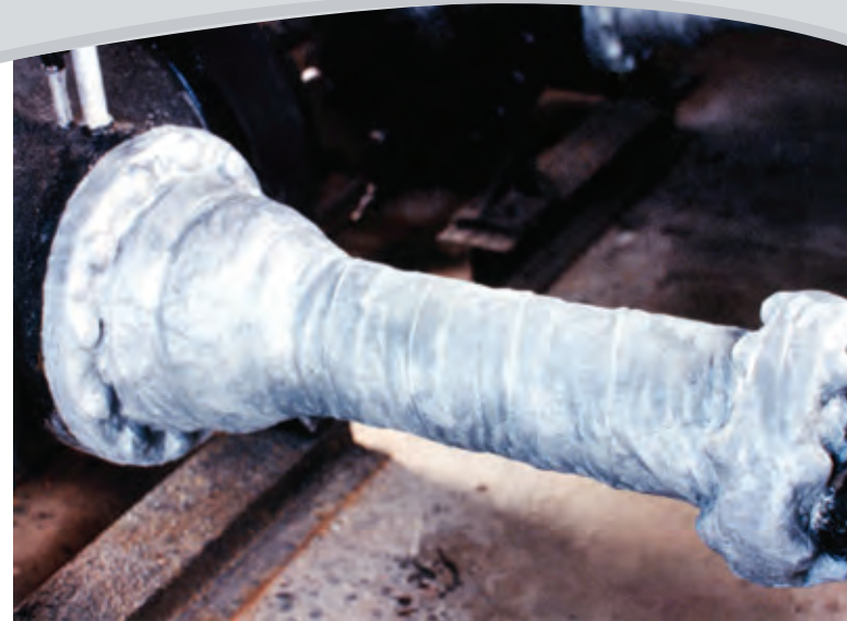
A sweating meter run pipe protected with Wax-Tape® #2A wrap demonstrates the wraps's ability to protect in wet conditions.
